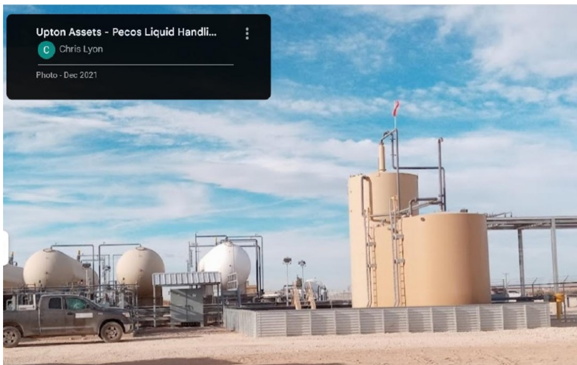
Fig 3: Original Tank Battery
